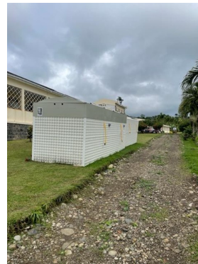
Figure 4: 3-phase septic tank at Mirabeau
